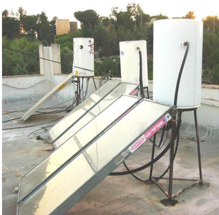
Fig. 2.6 : The common domestic water heating system in Gaza strip Source : (Wikipedia, 2011)
